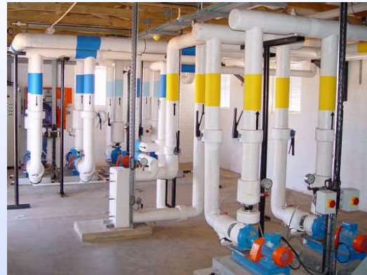
Facility Building & Services
